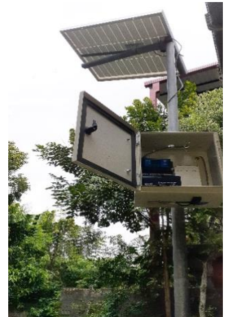
Fig.8. Installation with 50W solar panel
